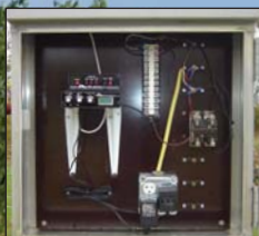
AR2 & AR2L Mounted in an outdoor enclosure with 110V lighting relay controls
